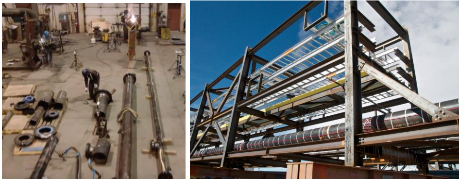
Organized Shop and Pipe Rack.
