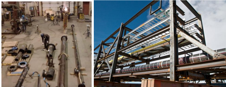
Organized Shop and Pipe Rack.
