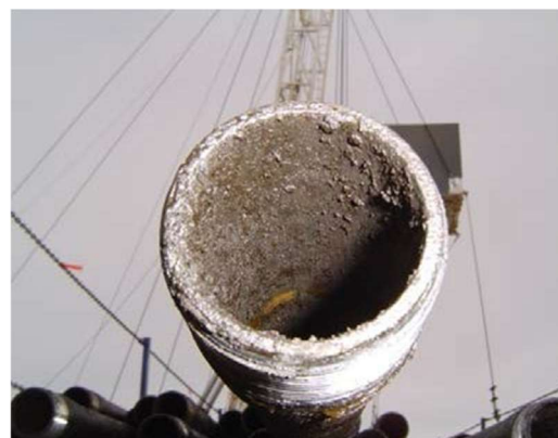
Scale containing NORM on service line
